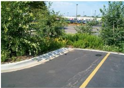
The sunken curb holds the edge of the asphalt pavement and lets water freely flow to the bioretention cell beside the 7sigma parking lot in Minneapolis, MN (USA)
